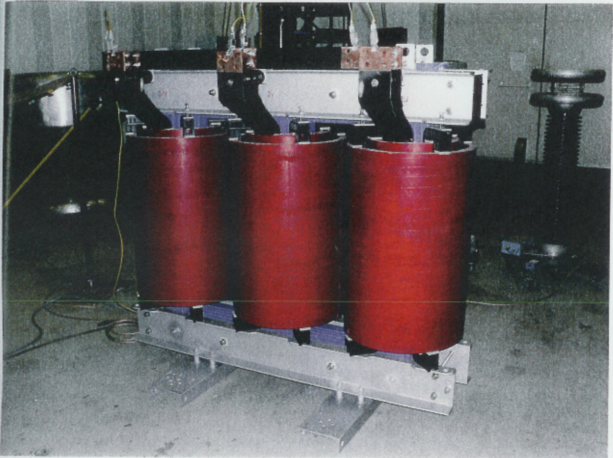
Photograph 2 Transformer seen from the low-voltage side
